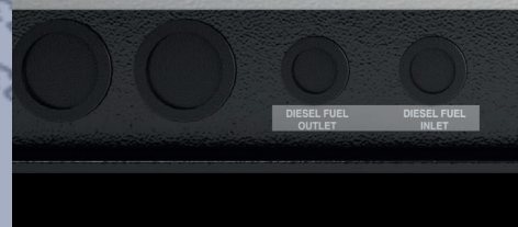
INPUT/OUTPUT FUEL PIPE
