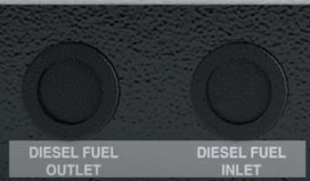
INPUT/OUTPUT FUEL PIPE
