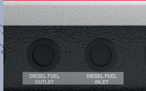
INPUT/OUTPUT FUEL PIPE
