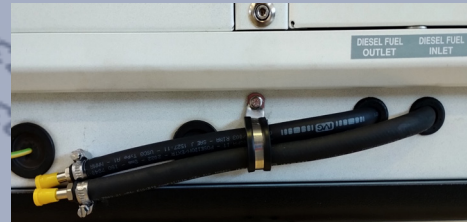
INPUT/OUTPUT FUEL PIPE
