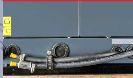
INPUT/OUTPUT FUEL PIPE
